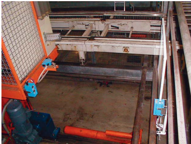
new optical data transfer-profibus and new laser distance measurement to the positioning
