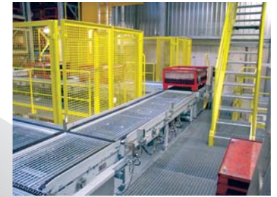
high rack warehouse with decentral frequency controller
