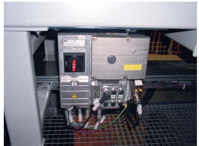
external field splitter of SEW
