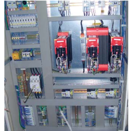
new on board S/R machine control cabinet
